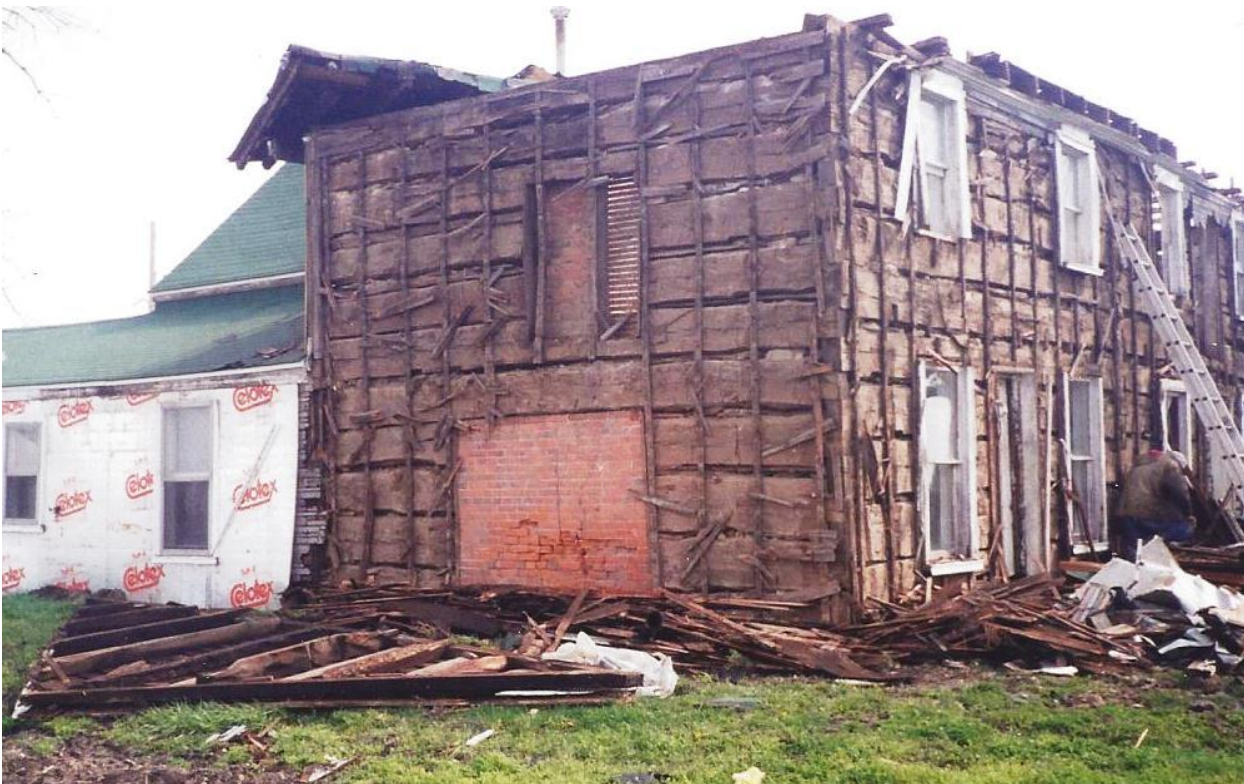
Modern inside brick chimney retrofit is exposed. Original wood chimney long-removed. Front & Rear hewn logs weigh 1,530 lbs each, which is why two-story log buildings were rarely built. Fireplace openings on 1 st & 2 nd floors are offset as each had separate, side-by-side flumes. Hewn logs are 20" x 6" X up to 20'.
